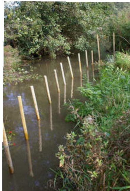
River narrowing 2, the first step. Perimeter of stakes on which hazel faggots are "impaled" to form the outer wall [11/10]
