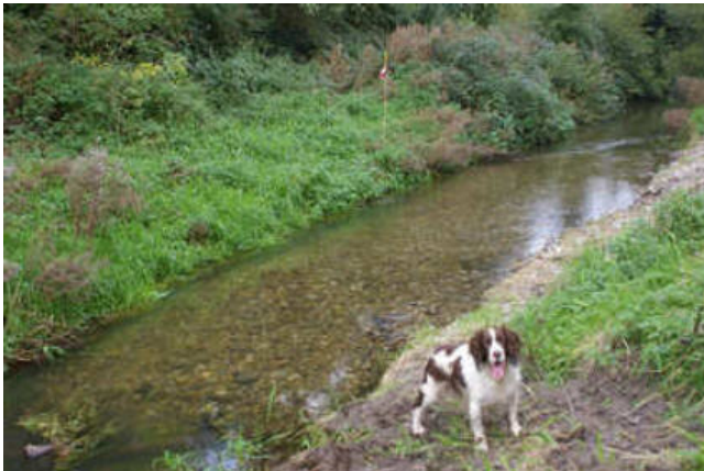
LWD 1, at head of riffle 2. Set into bank by digger, braced by posts and Wiring [16/10]
