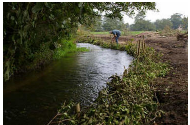
Protection of the re-profiled bank against erosion in flood until vegetation is re-established (technique as for river narrowing) [16/10]
