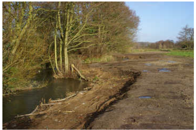
View 6 weeks after work completion. Shows the shape of the river revealed, the area of spoil coverage, and bank protection [07/12]
