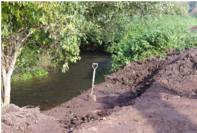
Re-profiling the river bank (the shovel is to clean the digger bucket!) [11/10]
