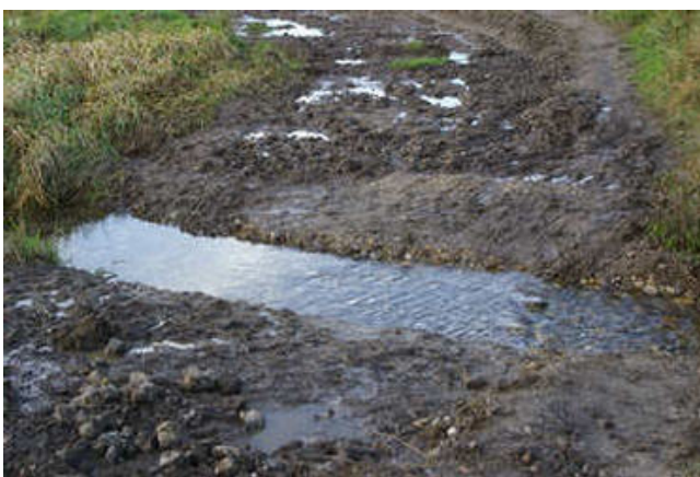
Final stages of re-instating side channel approaches; recovered large flint was used in cattle crossing 3 [07/12]
