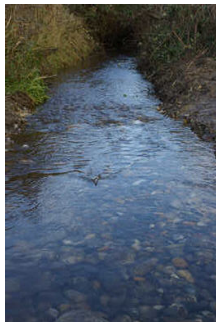
Small stone recovered was used to re-instate stream bed at the crossing, and Extend upstream and (shown) downstream [07/12]
